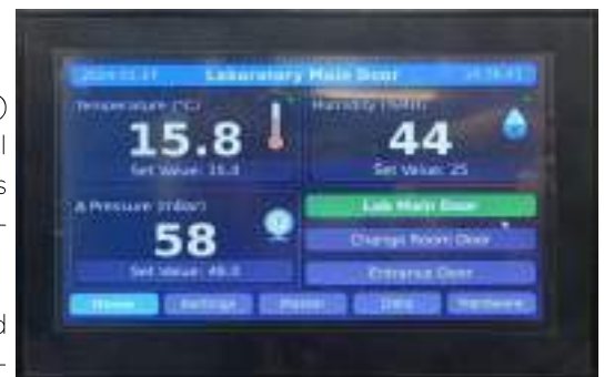
Touchscreen Controller with automatic Controlling of Temperature, Pressure & Humidity
